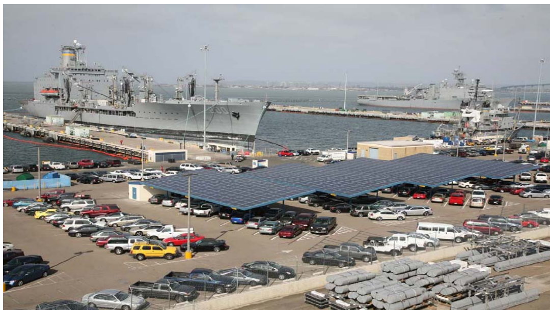
NAVAC Southwest Solar Carport in der San Diego Naval Bases
