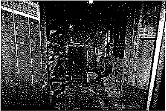
Local technique – chaudière bois
